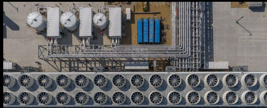
Rooftop Closed-Loop Liquid Cooling
